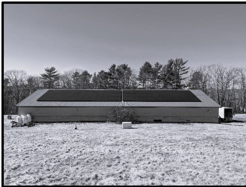
The Town's new solar array, located on the Community Hall!
